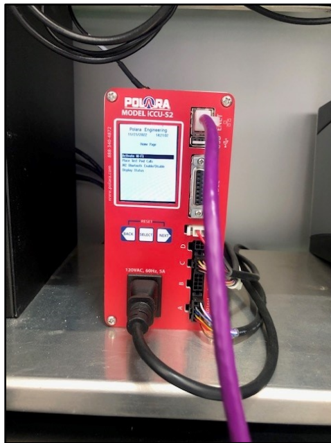
Accessible Pedestrian Push Button iCCU-S2 unit
