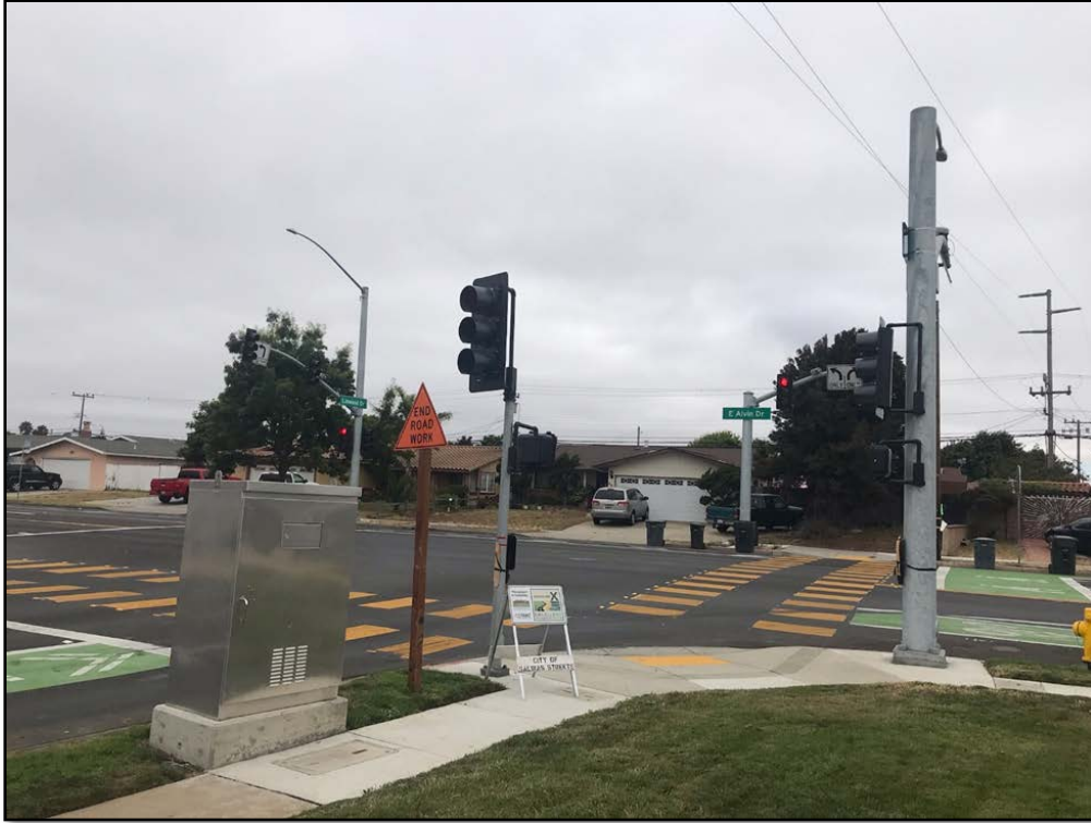
Construction Photo: Nearly Complete Signal at Alvin and Linwood with measure x signage
