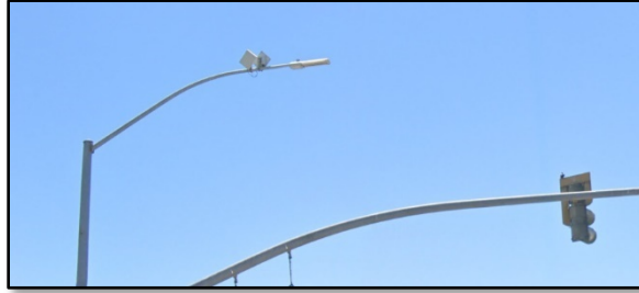
Radio installation at signalized intersections
