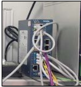
New Actelis Switch for communication to and from signalized intersections
