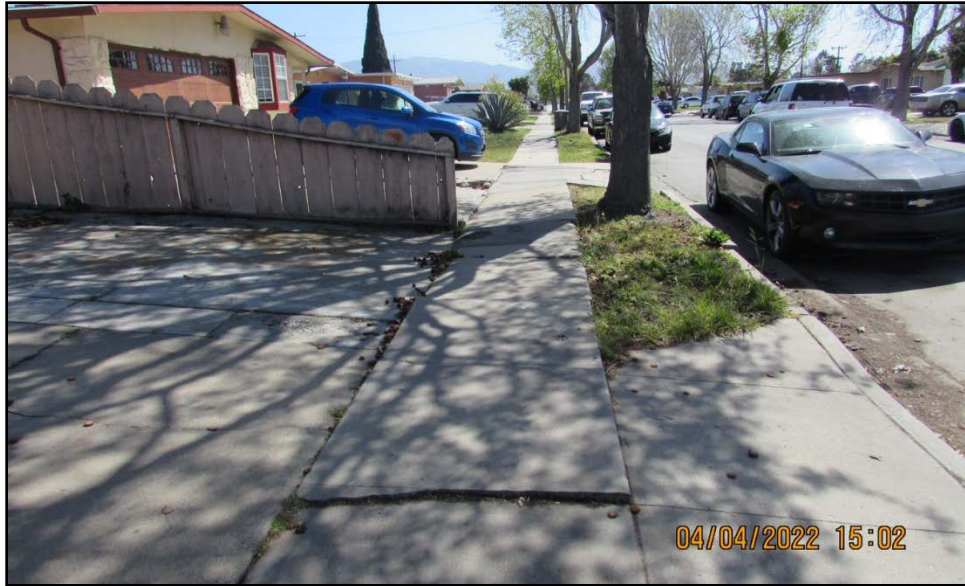
Before photo of S Filice St JOC Sidewalk Repair
