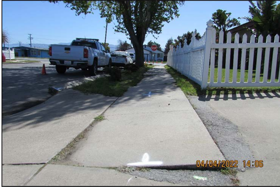
Before photo of S Filice St JOC Sidewalk Repair
