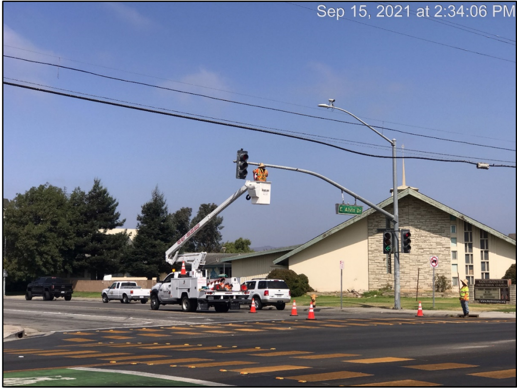
Construction Photo – Installation of mast arm signs at E Alvin Dr and McKinnon St
