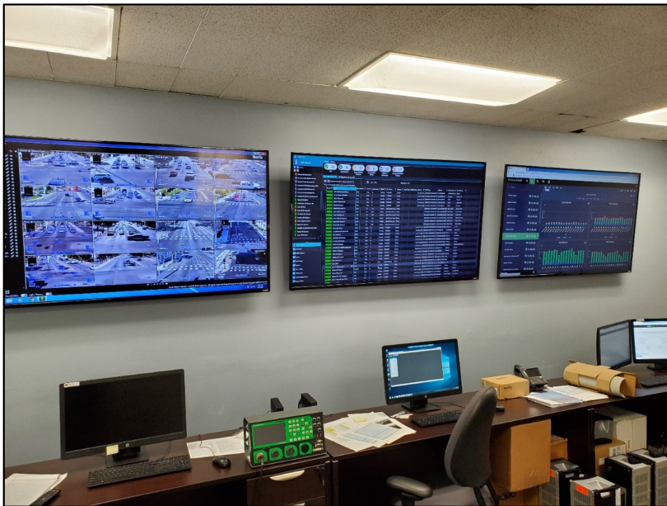
Traffic Signal Operations Monitored from the City's TOC.
