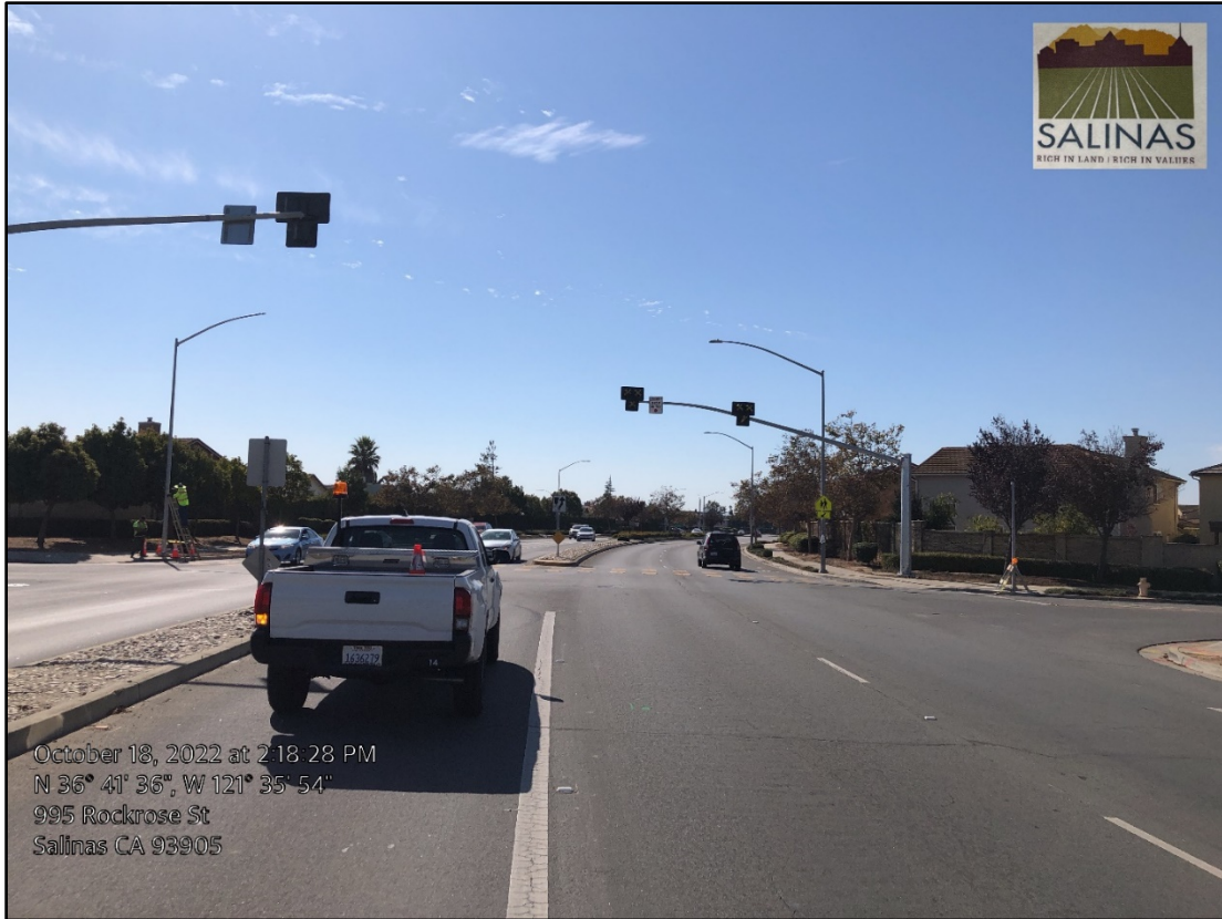
Construction Photo: Installing the Pedestrian Hybrid Beacon at Sanborn Rd and Buckhorn Dr
