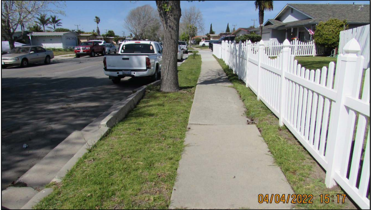
Before photo of S Filice St JOC Sidewalk Repair
