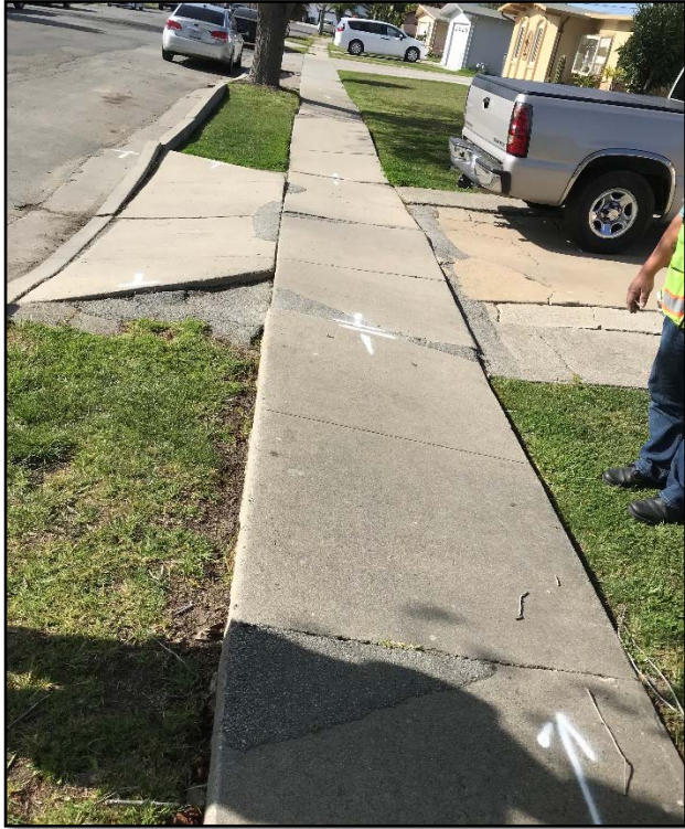
Before photo of S Filice St JOC Sidewalk Repair
