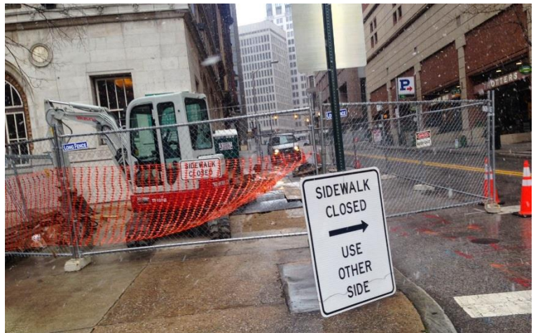
A practice that should be forbidden, i.e. a pedestrian path should be marked along the construction fence
