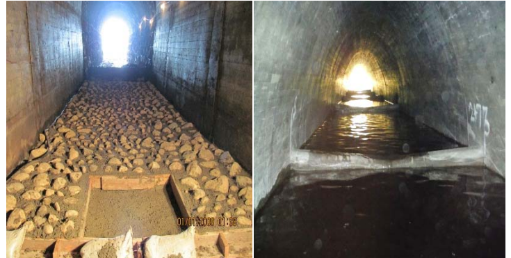
Facing upstream, southbound US 101 culvert fish passage at Tajiguas Creek along the Gaviota Coast in Santa Barbara County.
